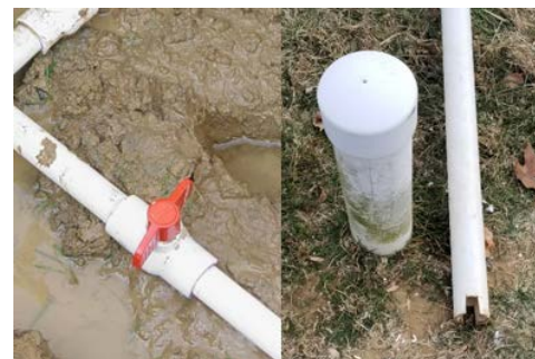
Shut-off valves can be very useful and a needed part of your water contingency plan.
